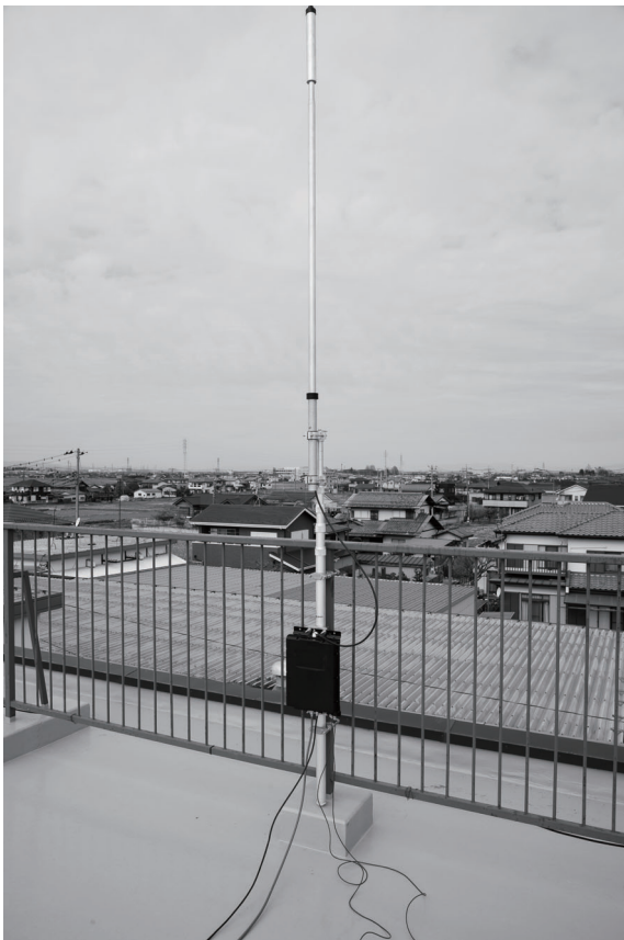
(Picture-1) Fixing the antenna mast (DAP600) at the support column of the hand rail, installing the element at the tip of the mast, fixing the ATU at the mast.
